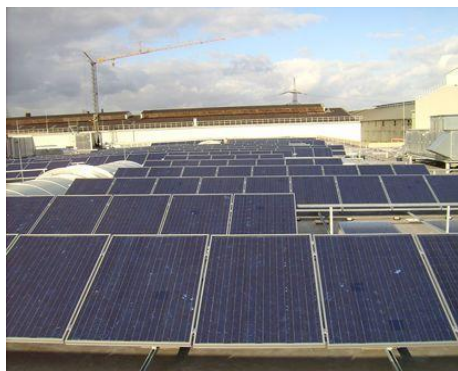
PV-panels in Gelsenkirchen
